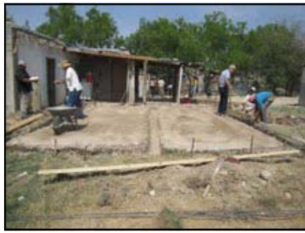
Above: Chuck Kinzler and David Manning start the foundation for a house in Piedras Negras at the end of March with the help of three workers from El Buen Pastor.
